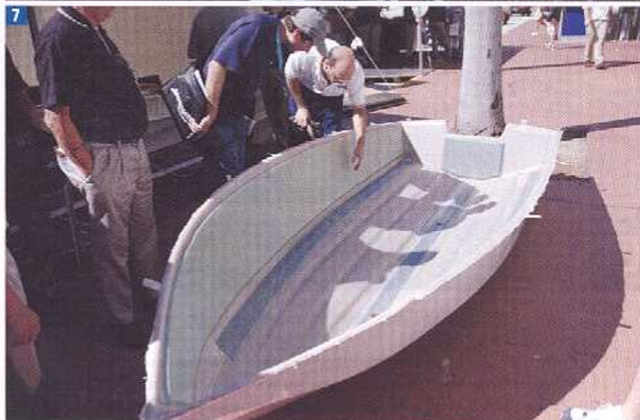
6 & 7 A demo at IBEX 2007 produced this dinghy hull. Using it is such a quick and simple process; and consumables are kept to an absolute minimum. The flow media used was supplied by Polynova, a combination of Hiflux 90 and Polybeam 703, and the core was Airex R63 80 foam. The resin came from Ashland.
